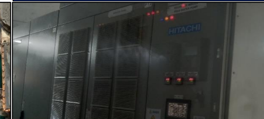
HT VFD for feed Pump
