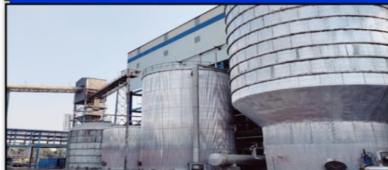
DDS technology digester
